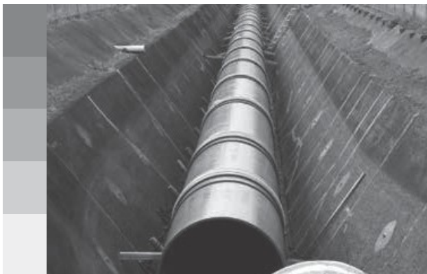
農業用水管 Agricultural Water pipes
